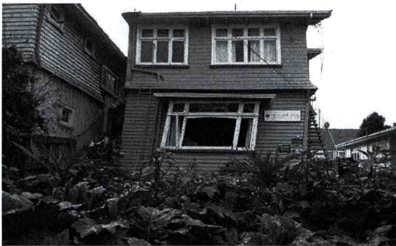
Damage to wooden structures.
