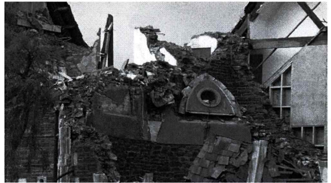
Damage after February 22 nd 2011
